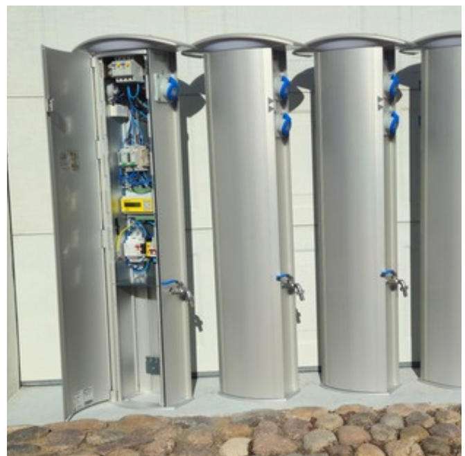
Pedestals from other providers, upgraded with our Emiko controller inside.
